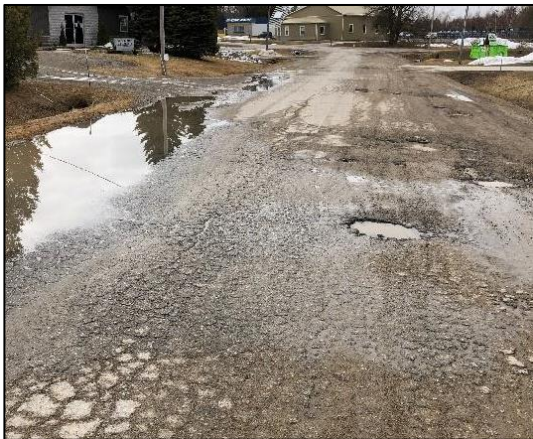
Figure 11-10: Poor Condition (PCR < 60)
