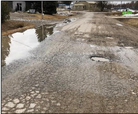
Figure 6-11: Poor Condition (PCR < 60)
