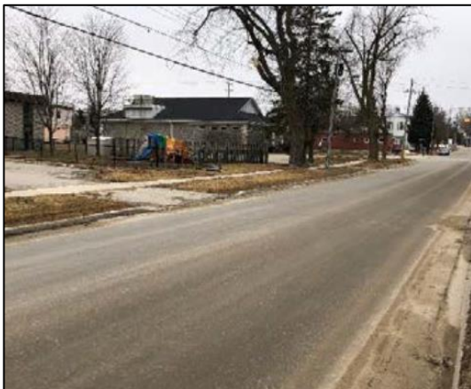
Figure 6-13: Good Condition (PCR 70 - 85)
